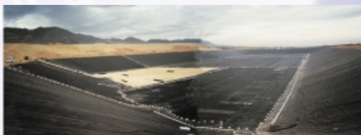
Panel extension and welding at the bottom. Distribution of final ballasting with concrete kerbs
