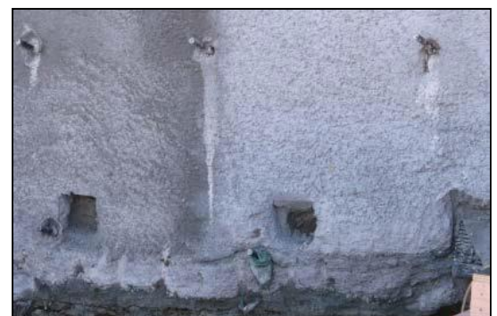
Megaflo® drainage holes through shotcrete
