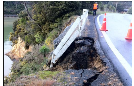
Slip prior to repairs
