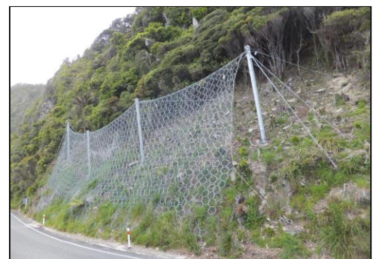
Completed 3000kJ Hybrid Fence
