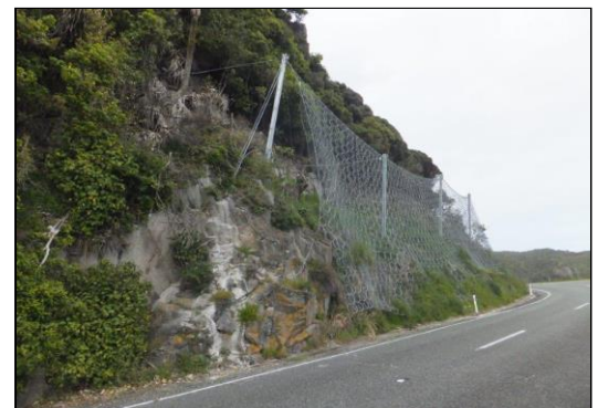
Completed 3000kJ Hybrid Fence
