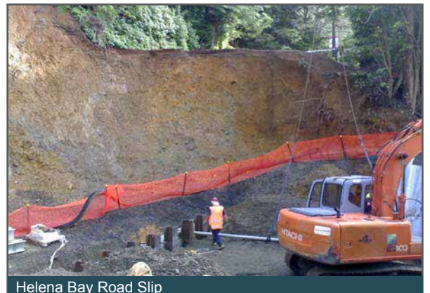
Helena Bay Road Slip
