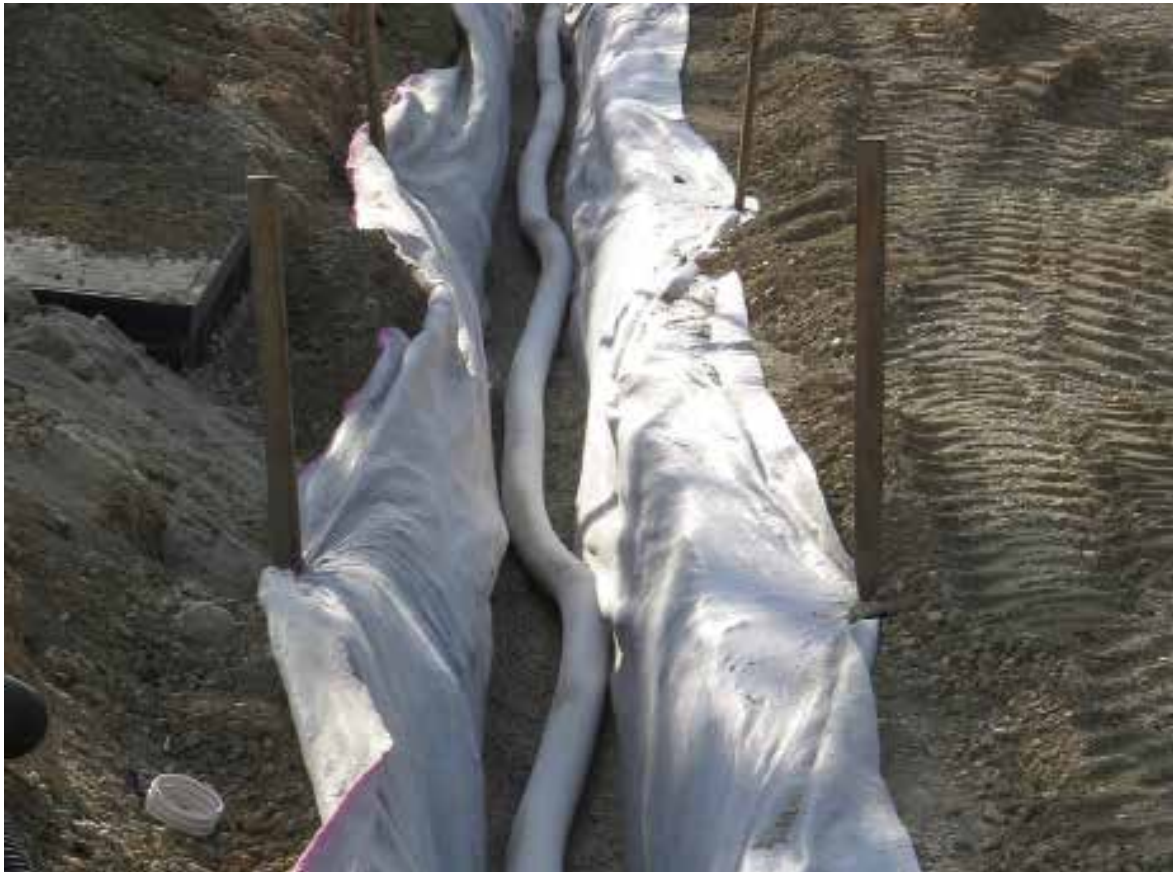
Greenflo Filter Sock on perforated round pipe in Bidim geotextile wrapped trench
