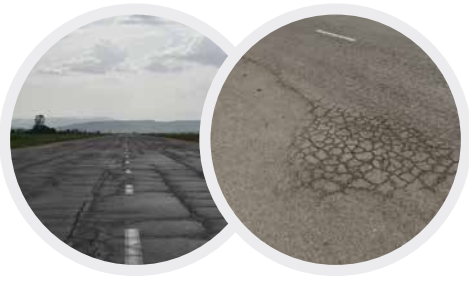
Example of cracking for area-wide repairs
