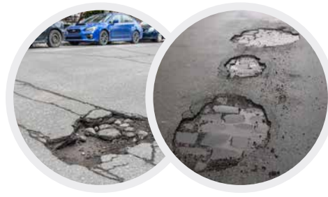
Example of cracking for local repairs
