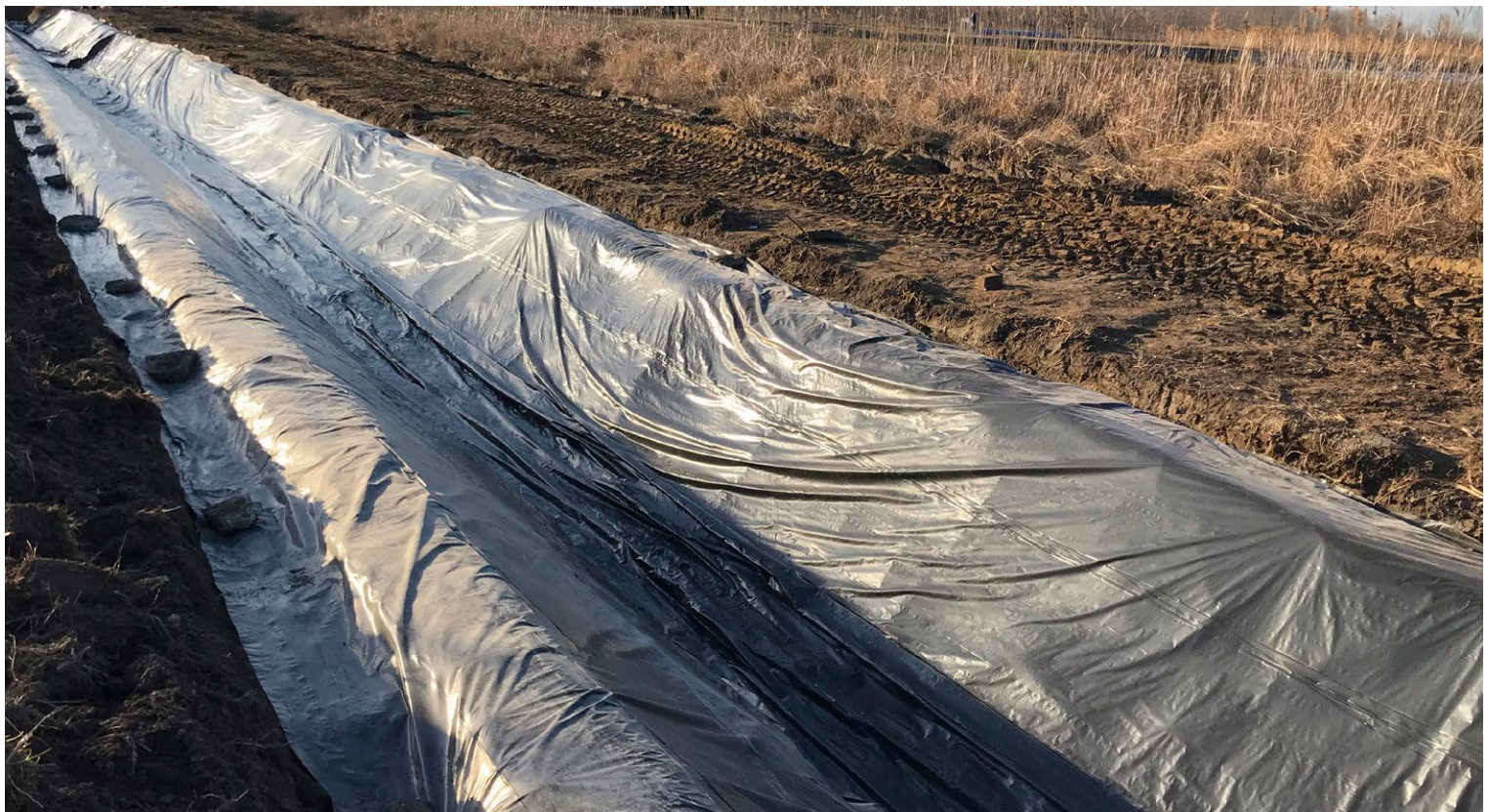
Hydrated CCX-M™ covered with plastic sheeting to maximise curing conditions during low temperatures
