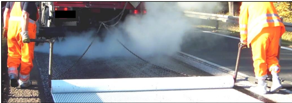
Picture 4: Installation with traverse and adjust bars directly after spraying the bond coat
