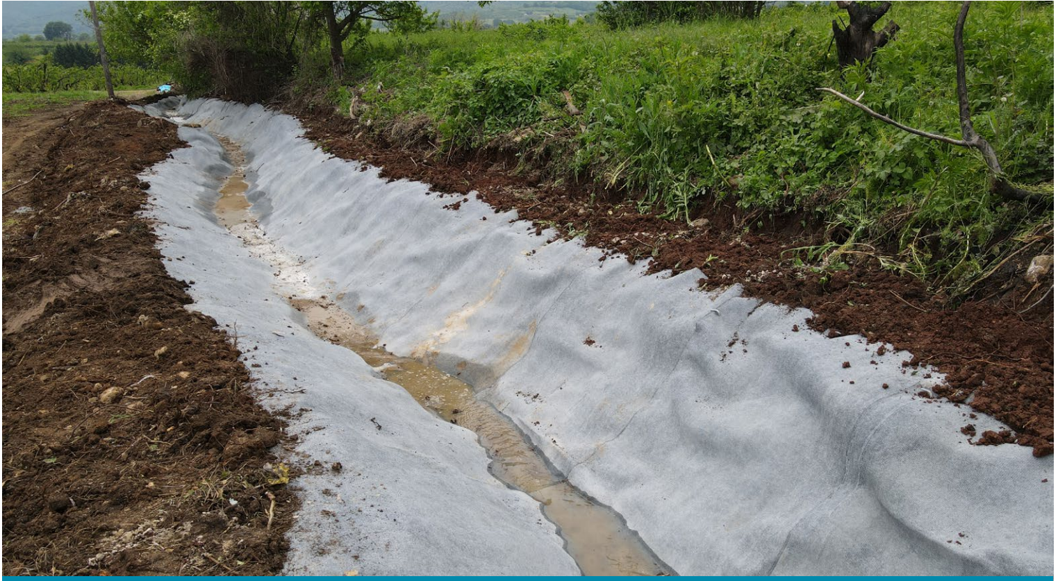
Completed CCX-M™ Installation
